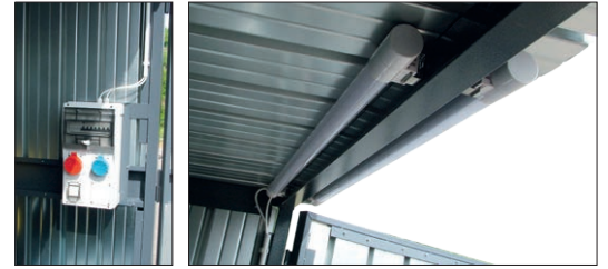
Electrical system And lighting
